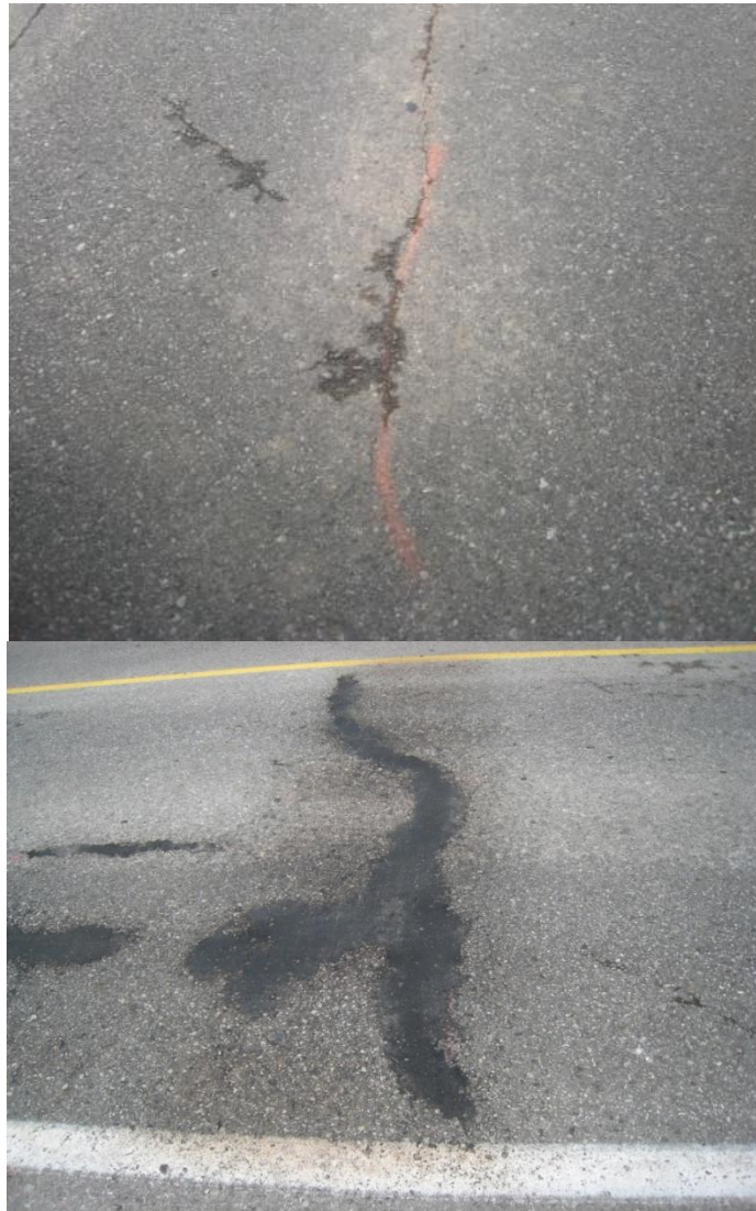
Figure 4 – Before and After Photos of Crack Repairs on Bleams Road Using Infrared Heating
