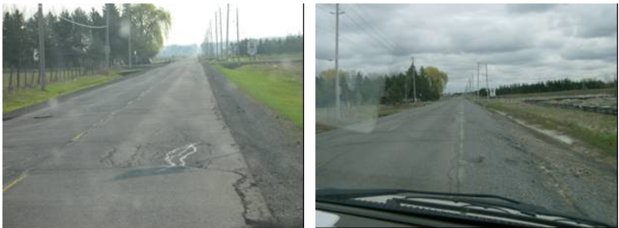
Figure 3: Edge Cracking, Pre and Post Construction (left and right respectively)
