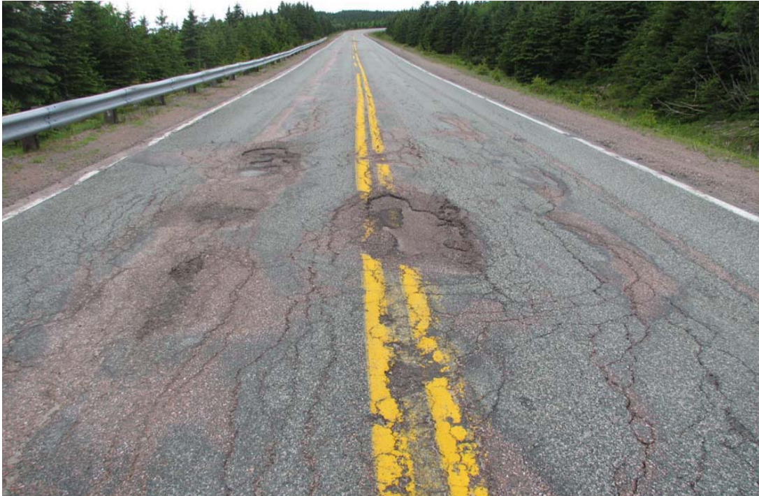
Figure 5 Pavement with a PCI of 43
