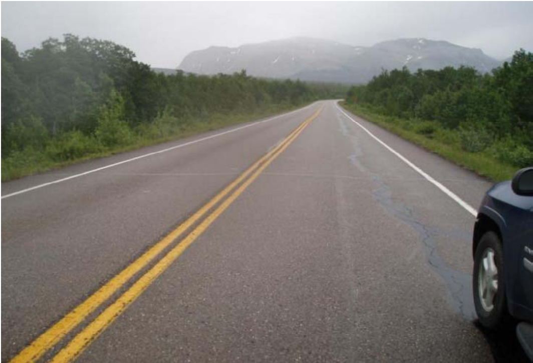
Figure 3 Pavement with a PCI of 64
