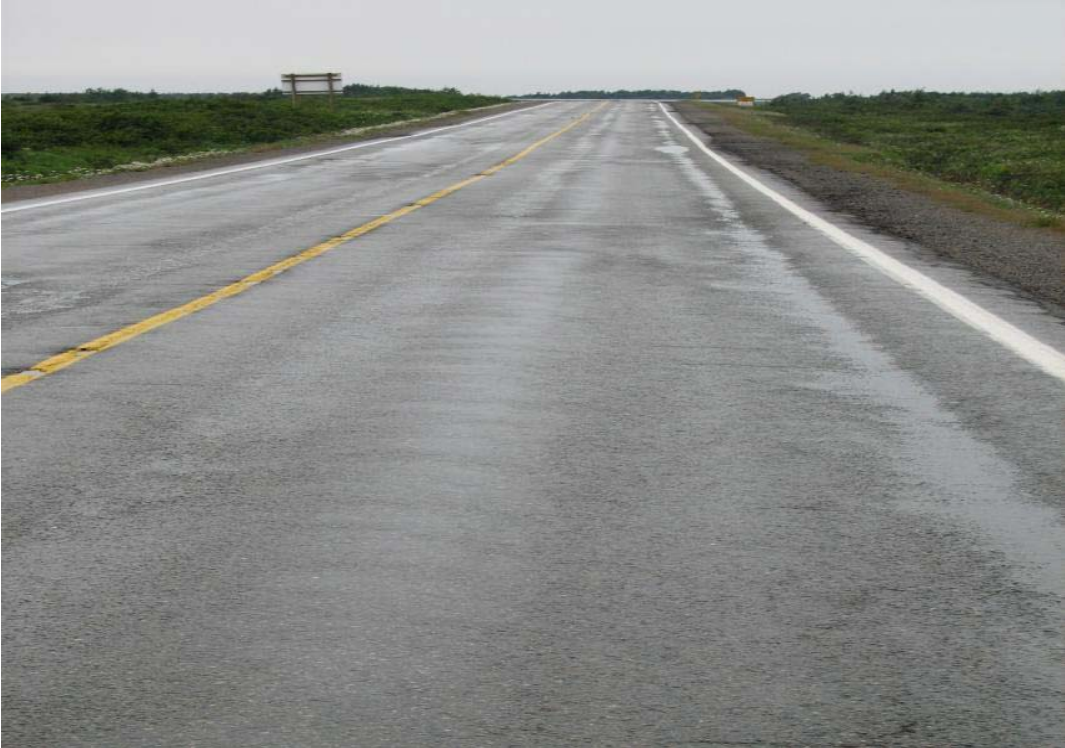
Figure 4 Pavement with a PCI of 58
