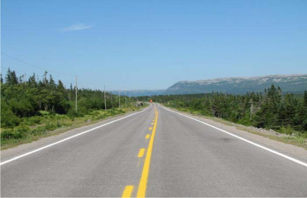
Figure 2 Pavement with a PCI of 71
