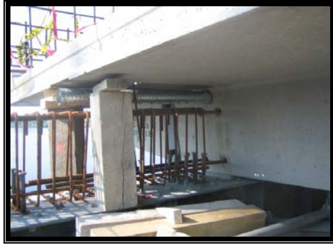
Figure 4: Composite Action between the Precast Deck and either the Plate Girder Top Flange or the deck Truss Top Chord.
