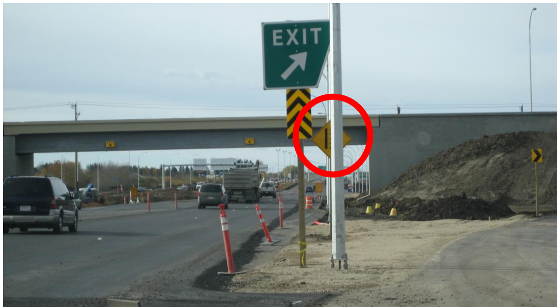
Figure 5: Example of poor field-fitting of signs (obscured Lane Ends sign)
