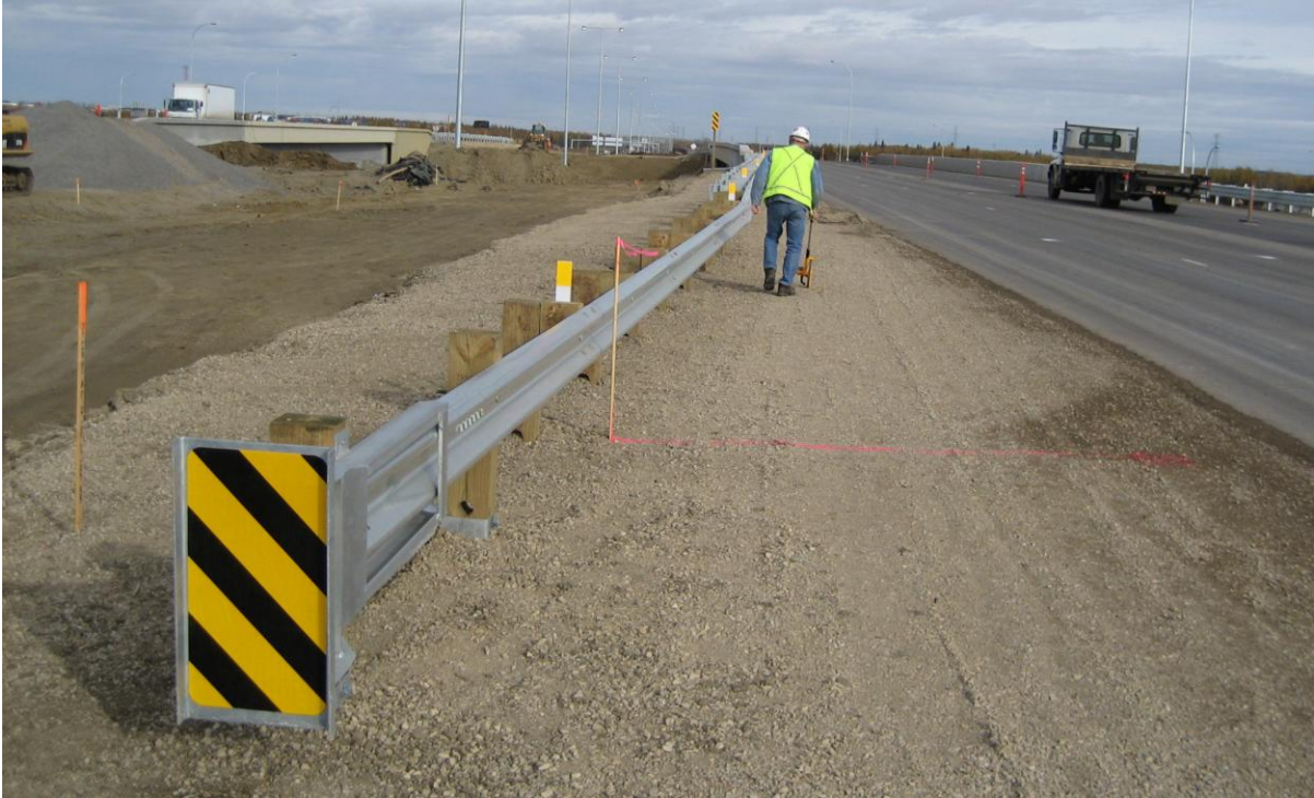
Figure 12: EAGRT installed with excessive flare
