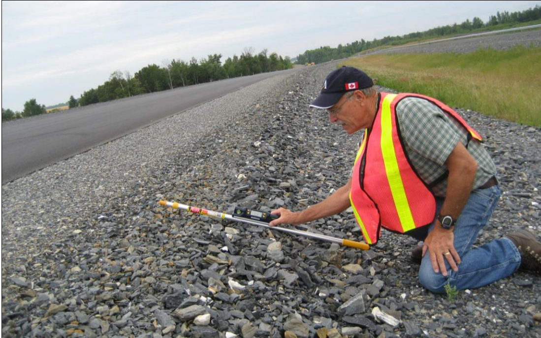
Figure 9: Improper grading resulting in non-recoverable foreslope
