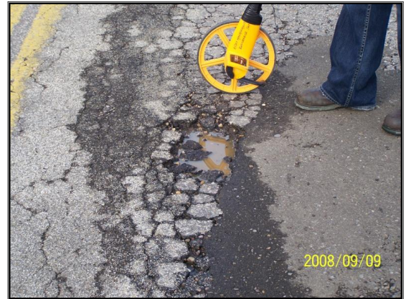
Figure 11 – Extreme Alligator Cracking.
