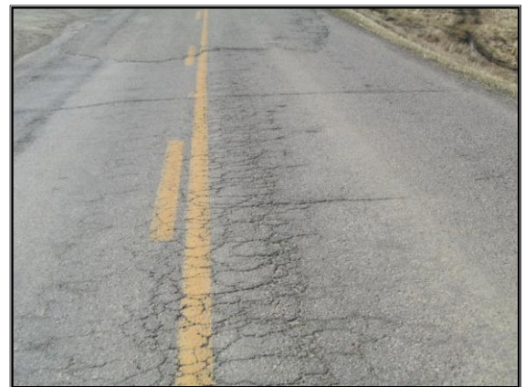
Figure 12 – Moderate Alligator Cracking.
