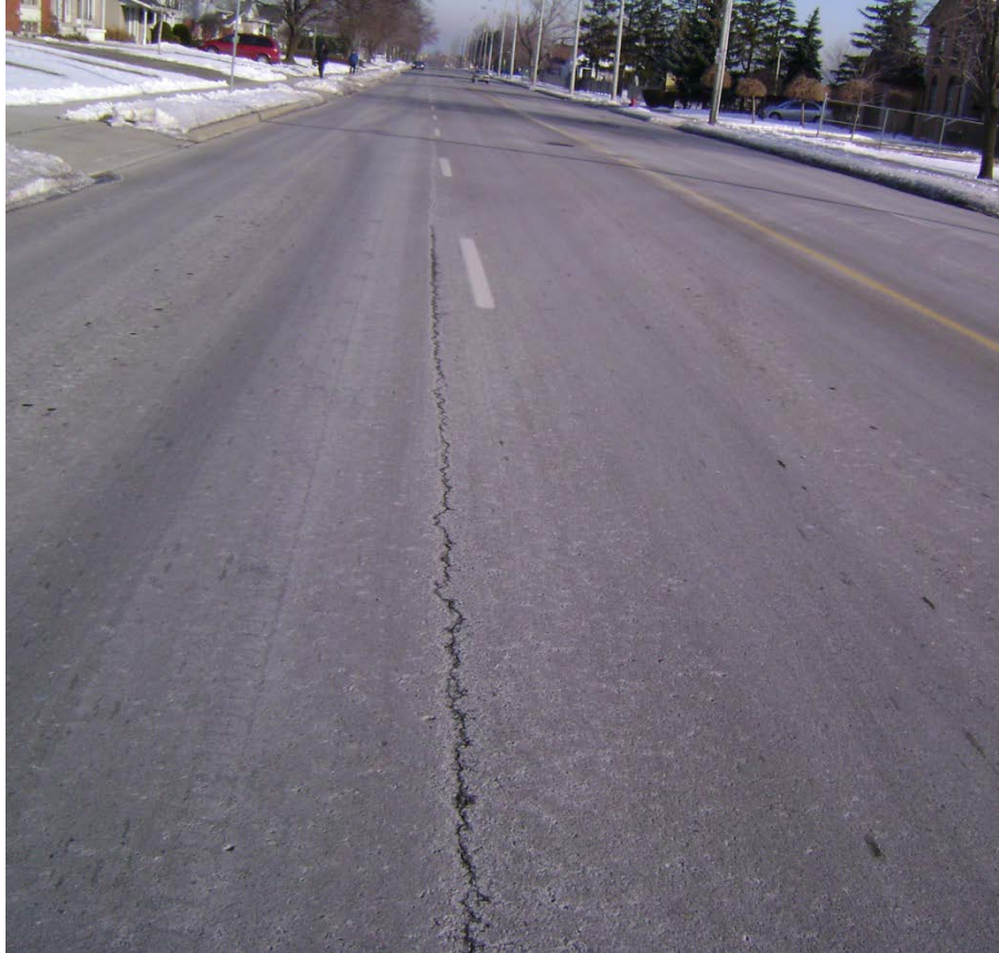
Figure 1: Example of poor longitudinal joint in newly constructed pavement.
