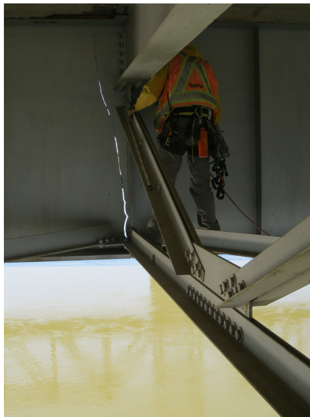
Figure 6 Crack location at connection
