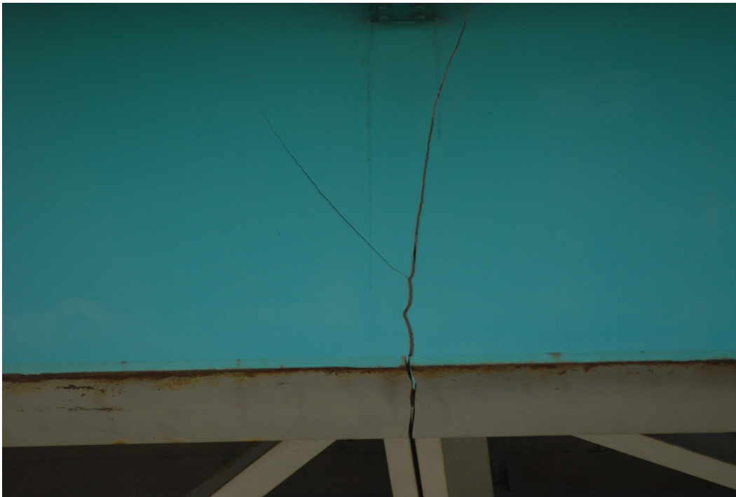
Figure 5 Closer view of crack bi-furcation
