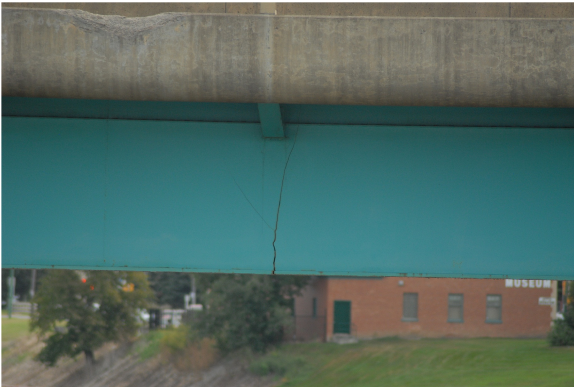
Figure 4 Crack showing bi-furcation
