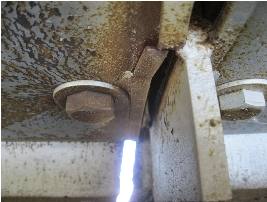
Figure 9 Crack surface and weld fracture (underside of gusset shown)
