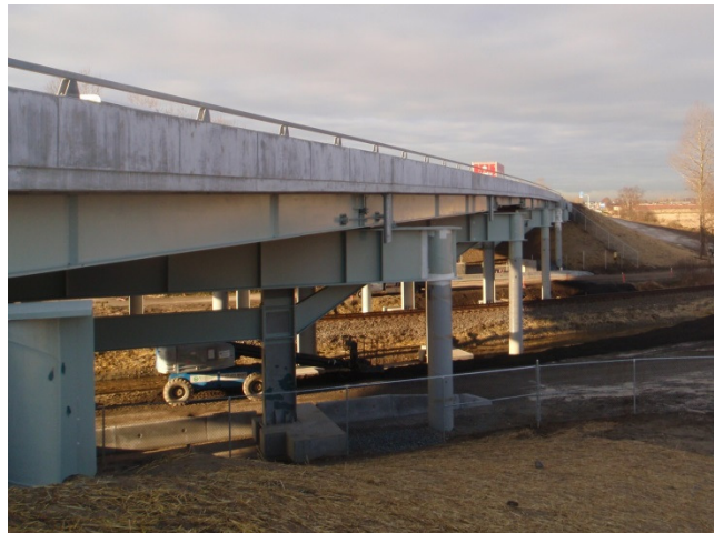
Figure 6 – Photo of the "Catcher" frame system
