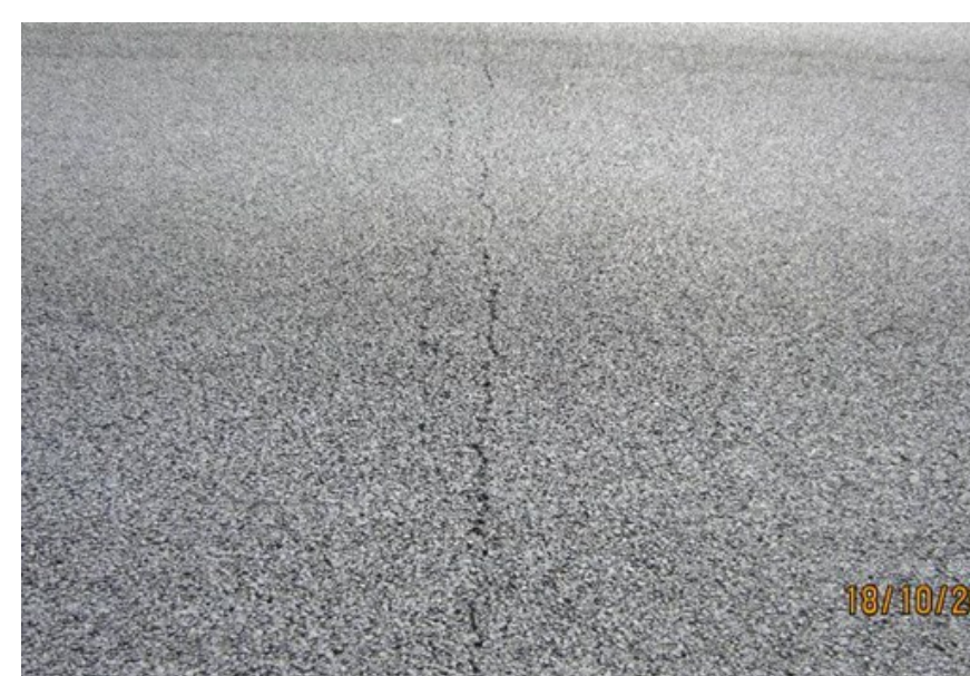
Section B - Transverse Crack
