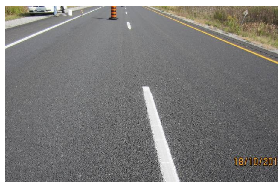
Section A - Centreline Joint is Intact
