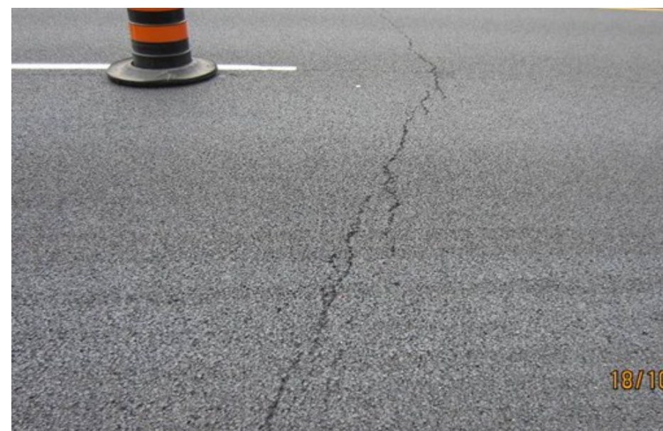
Section C - Transverse Crack
