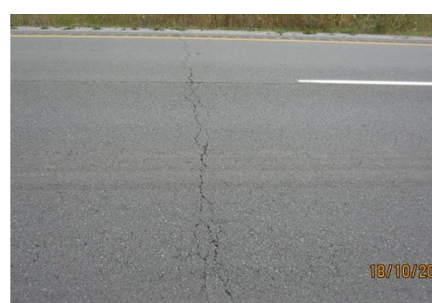
Control Section E - Transverse Crack
