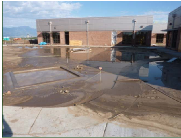
Figure 8. Clogged pavement due to lack of adequate protection during construction.
