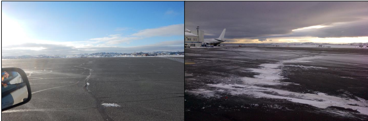
Figure 3 – Surface Distresses/Settlement Associated with Underlying Ice Wedges
