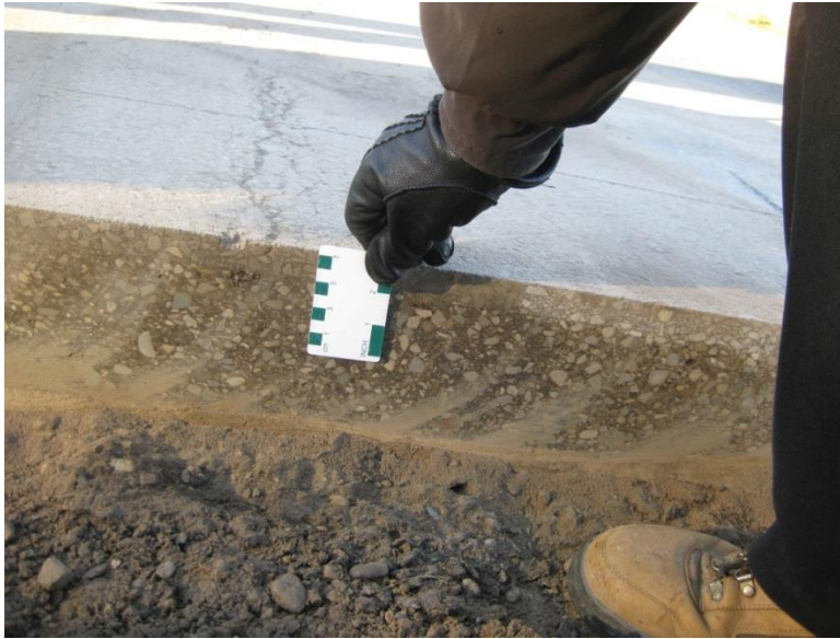
Photograph12 The crack in the investigated pavement was observed only in the surface course [LU, 2014]
