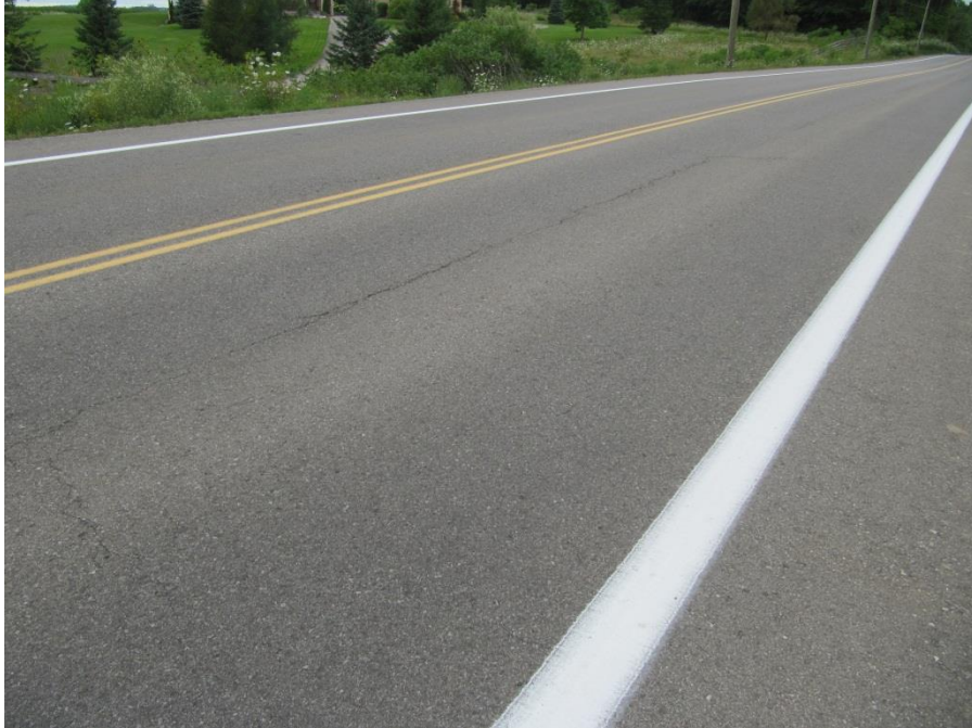
Photograph 4 Midlane cracking on Trussler Road [VH, 2014]
