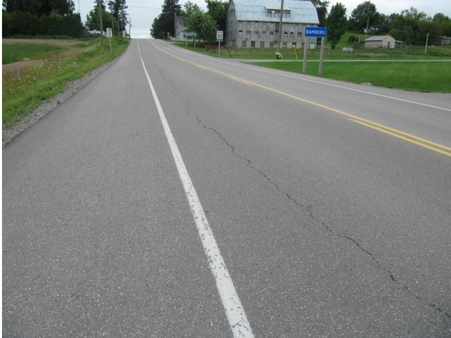
Photograph 6 Midlane cracking on Moser Young Road [VH, 2014]
