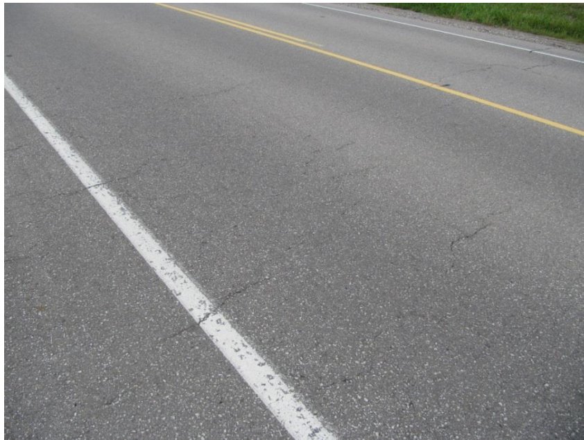
Photograph 7 Check cracking on Moser Young Road [VH, 2014]
