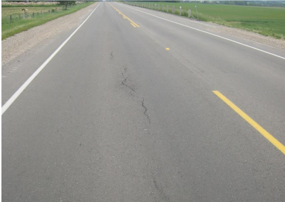
Photograph 1 Midlane cracking of a 6 months old pavement on Bleams Road constructed in 2009 [LU, 2010]
