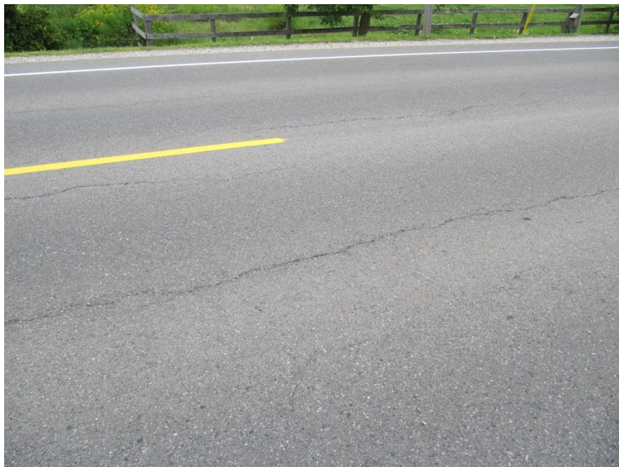
Photograph 3 Midlane and longitudinal cracking on Katherine Street [VH, 2014]
