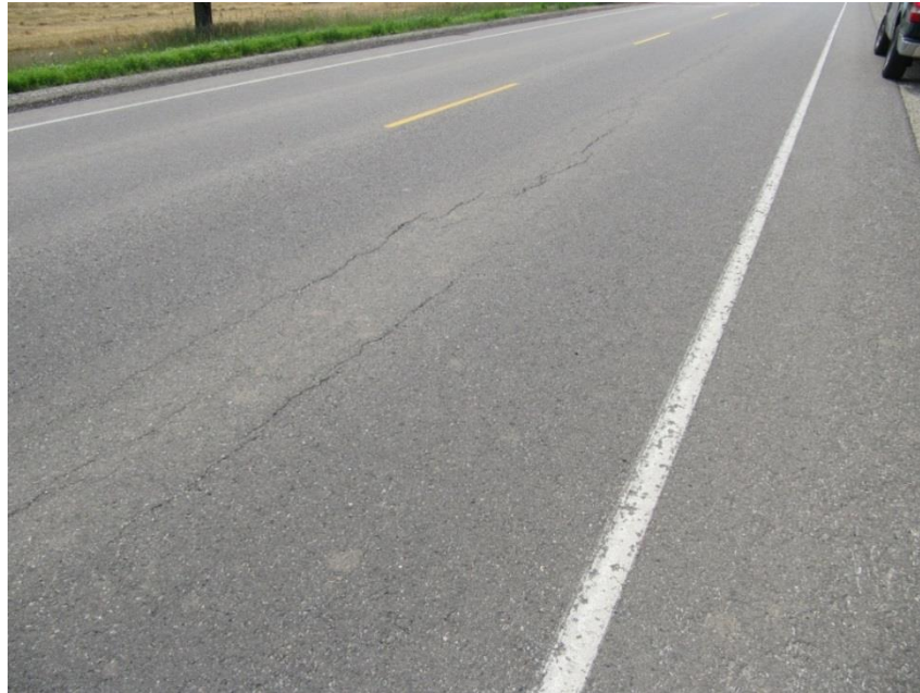
Photograph 2 Multiple midlane cracks on Katherine Street [VH, 2014]
