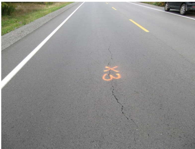
Photograph 9 Cracking on Portage Road constructed in 2013 [VH, 2014]
