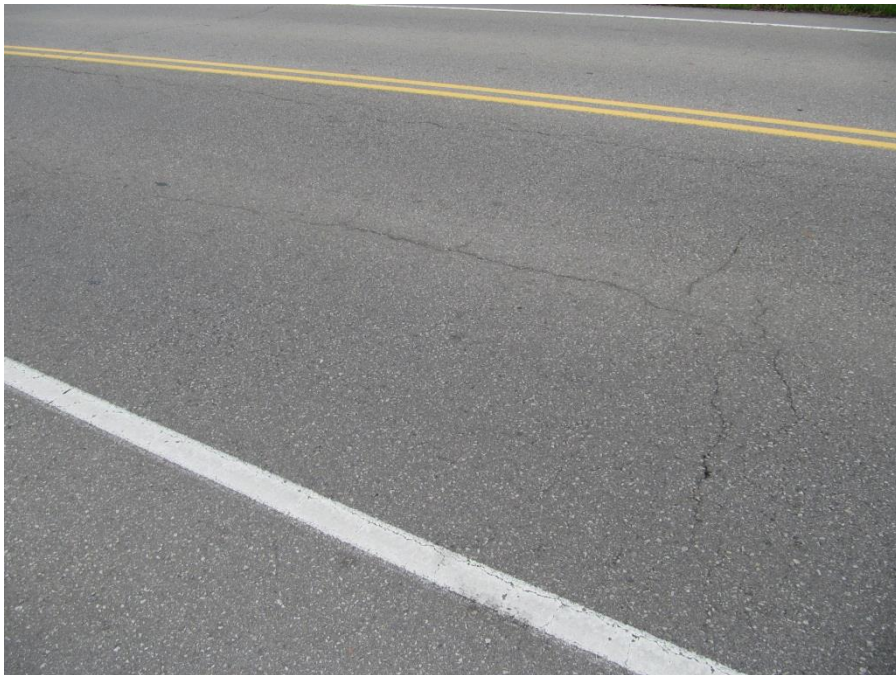
Photograph 5 Midlane, longitudinal and check cracking on Swan Street [VH, 2014]
