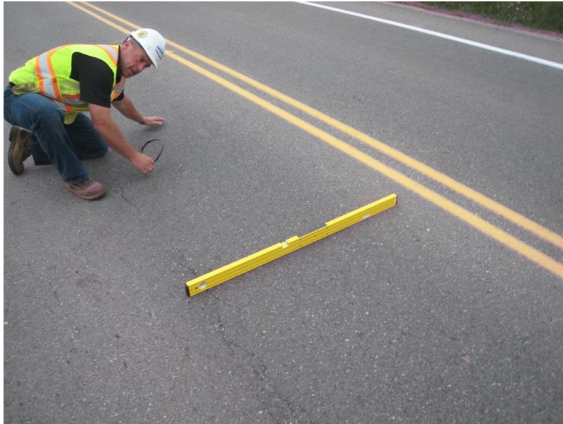
Photograph 10 No rutting was observed on the 2 years old cracked pavement [LU, 2014]
