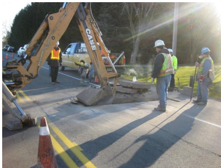
Photograph 11 Cutting asphalt slab as part of the failure investigation on 2 year old pavement [LU, 2014]
