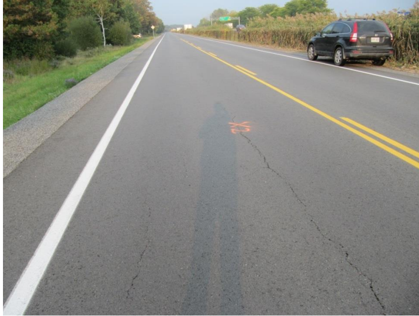
Photograph 8 Cracking on Portage Road constructed in 2013 [VH, 2014]
