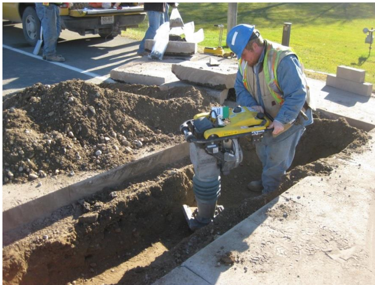
Photograph 13 Reinstatement of the granular base layer after checking its quality and obtaining samples for laboratory testing [LU, 2014]
