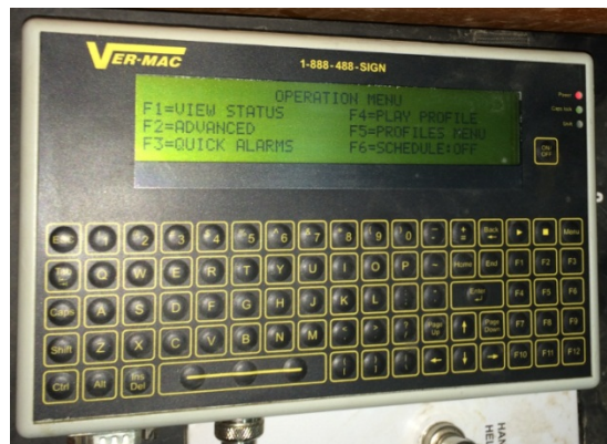
Figure V: Controller box located within the unit on Leg #1
