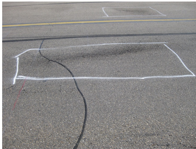
Figure 3 – Shear Cracking and Shoving on Runway at Edmonton International Airport
