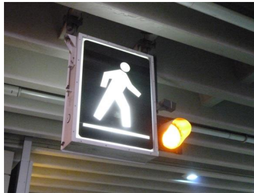
Figure 5.7 – Backlit Overhead Pedestrian Sign
