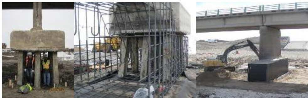
Figure 4 – Excavation Complete Beneath Pier (left), Reinforcing Steel for New Pier Footings (centre), Completed Pier Footing (right)
