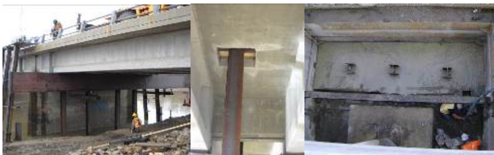
Figure 7 – Steel Support for Driving of New Piles (left), New Piles Driven Through Existing Deck (centre), Partial Concrete Tremie Plug for New Foundation (right)
