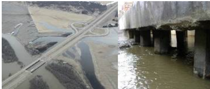
Figure 6 – TCH 1W During 2011 Flood (left), Exposed Piles Due to Scour at Pier SU.5 (right)
