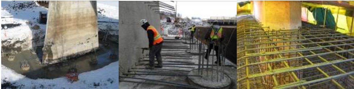
Figure 15 – Drilled Shaft Caissons for Footing (left), Anchoring Reinforcing Into Existing Pier (centre), Pier Footing Reinforcing (right)
