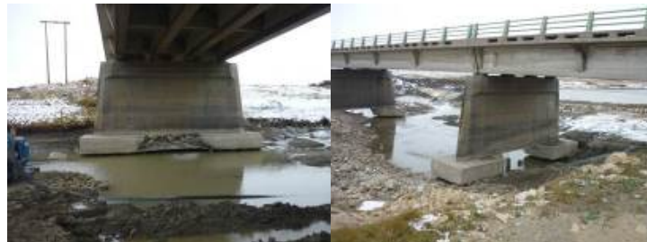
Figure 2 – Scouring Beneath Bridge Piers
