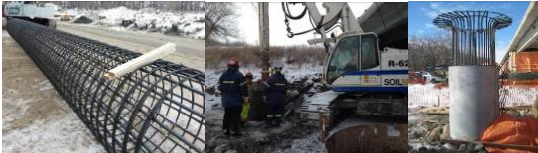
Figure 11 – Reinforcing Steel for Drilled Shaft Caisson (left), Drilling of Caisson, Metalized Steel Jacked Caisson and Reinforcing Steel (right)
