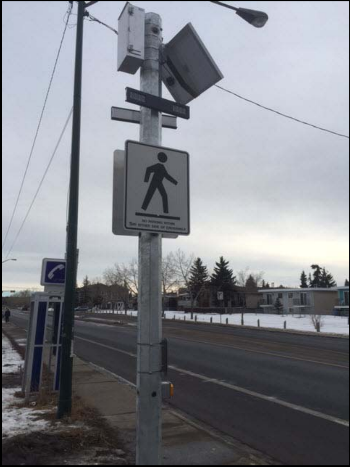
Figure 9: New RRFB installation on Bowness Rd NW as part of Phase 2 Pilot). Please note - The flashers are placed above the sign as opposed to below the sign in previous installations)
