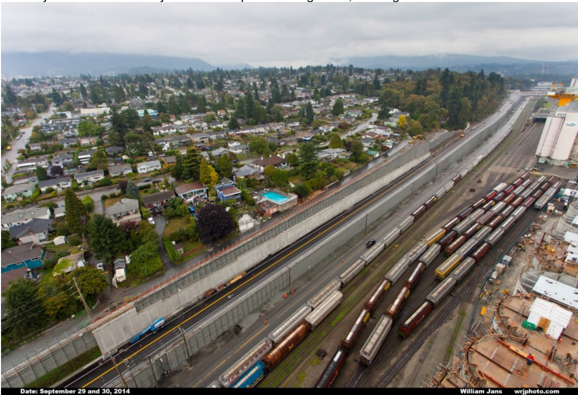
Low Level Road Corridor, after: A multi-tiered retaining wall system was implemented along the corridor to grade-separate motorists, pedestrians, cyclists, and rail traffic away from one another.
