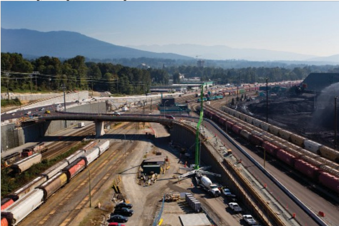
Port access, after: The Neptune/Cargill Overpass replaces the at-grade rail crossing with a unique
