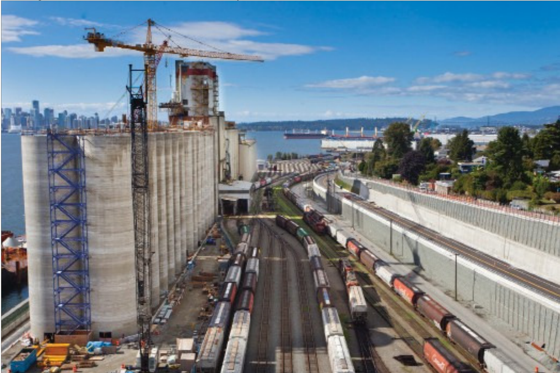
West end, after: New rail tracks, grade-separated from the laneway, increase port operational capacity while addressing safety issues and traffic challenges along the heavily-used Low Level Road Corridor
