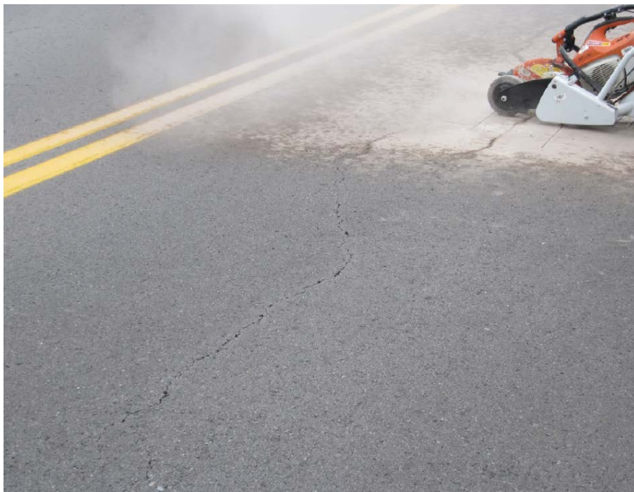
Photograph 15 Premature asphalt cracking on 6 months old pavement.
