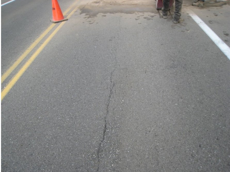
Photograph 14 Premature asphalt cracking on 2 years old pavement.
