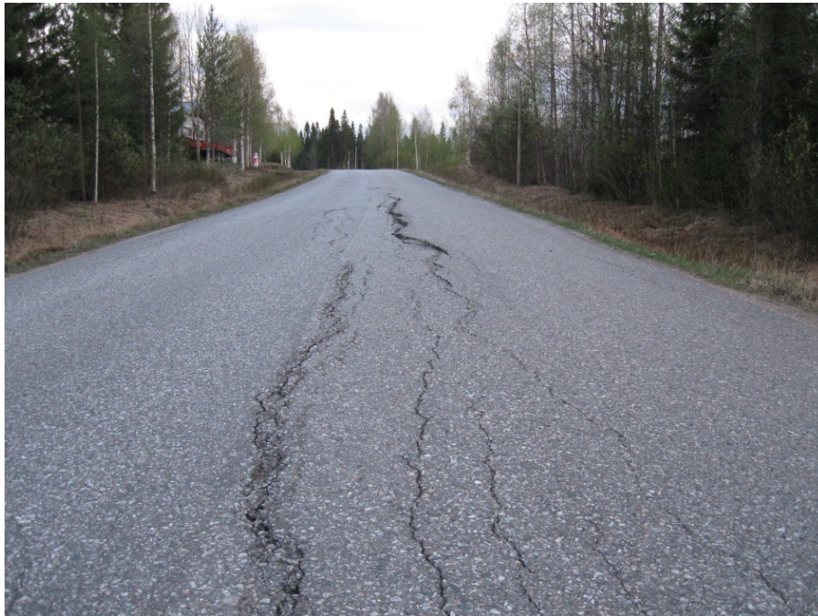
Photograph 12 Severe cracking on a rural pavement due to frost heaving.
