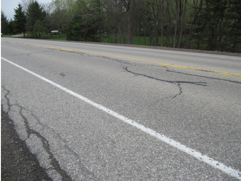
Photograph 3 Centerline, edge and localized alligator cracking in 19 years old cold in-place recycled pavement.
