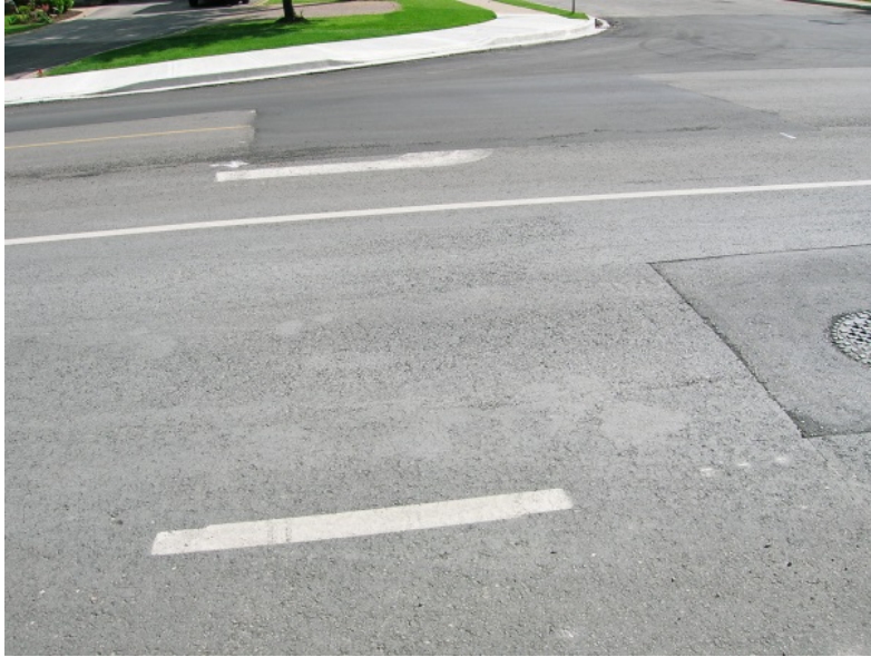
Photograph 8 Raveling and cracking of new binder course that incorporated very high content of RAP.
