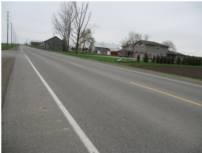
Photograph 4 Excellent current condition of 5 years old re-recycled with foamed asphalt stabilization pavement.
