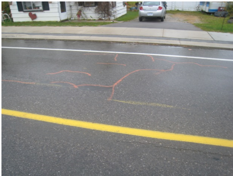
Photograph 9 Cracking of new binder course that contained high percentage of RAS.
