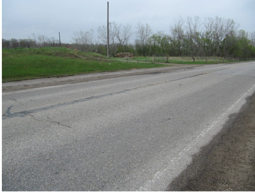
Photograph 1 Low severity joint and transverse cracking on 18 years old cold in-place recycled pavement. The overall condition is good.
