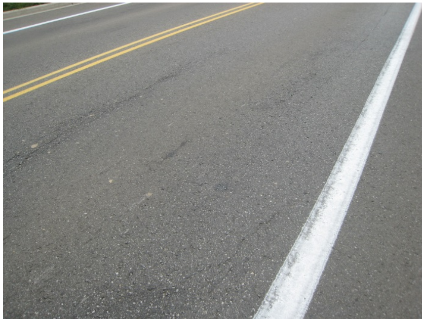
Photograph 13 Premature asphalt cracking on 2 years old pavement.
