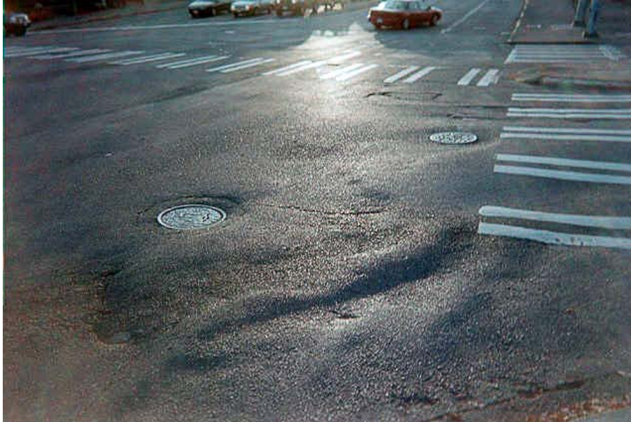
Photograph 11 Frost heaving deformation at an intersection in a vicinity of a manhole.
