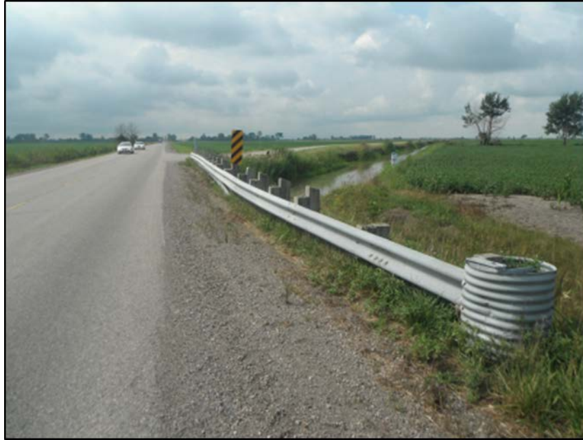
Figure 11 Entrance Conflict at Roadside Safety System Departure
