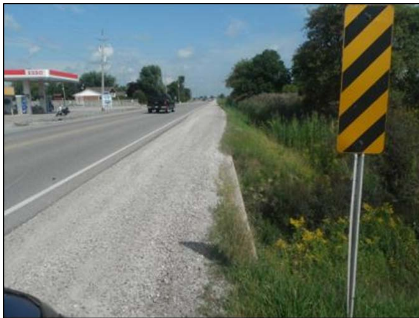
Figure 8 Fully Unprotected Roadside Hazard
