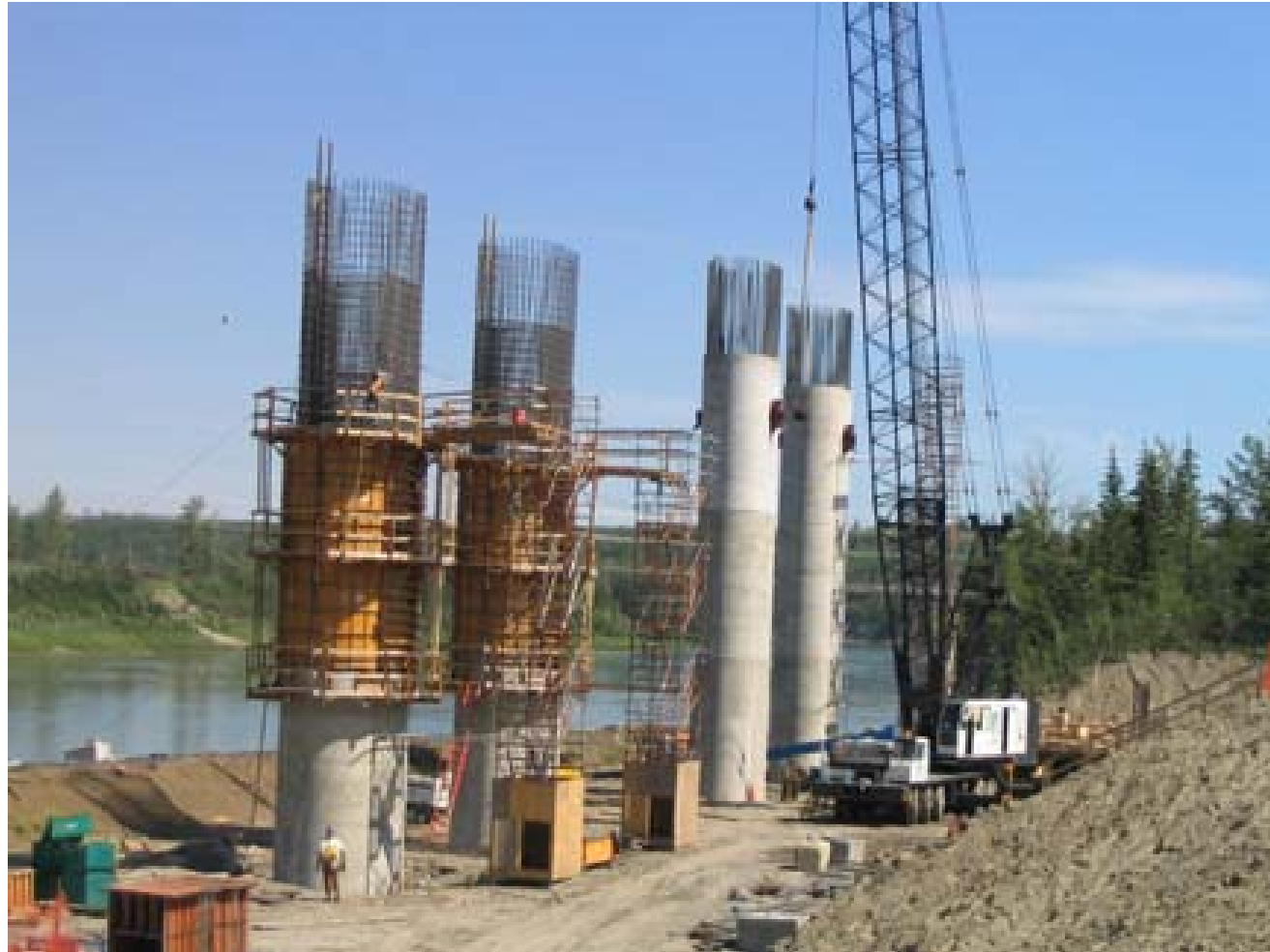
Figure 9: NBL Pier Shafts Completed and Preparing to Pour Second Lift on the SBL Pier Shafts at Pier 3
