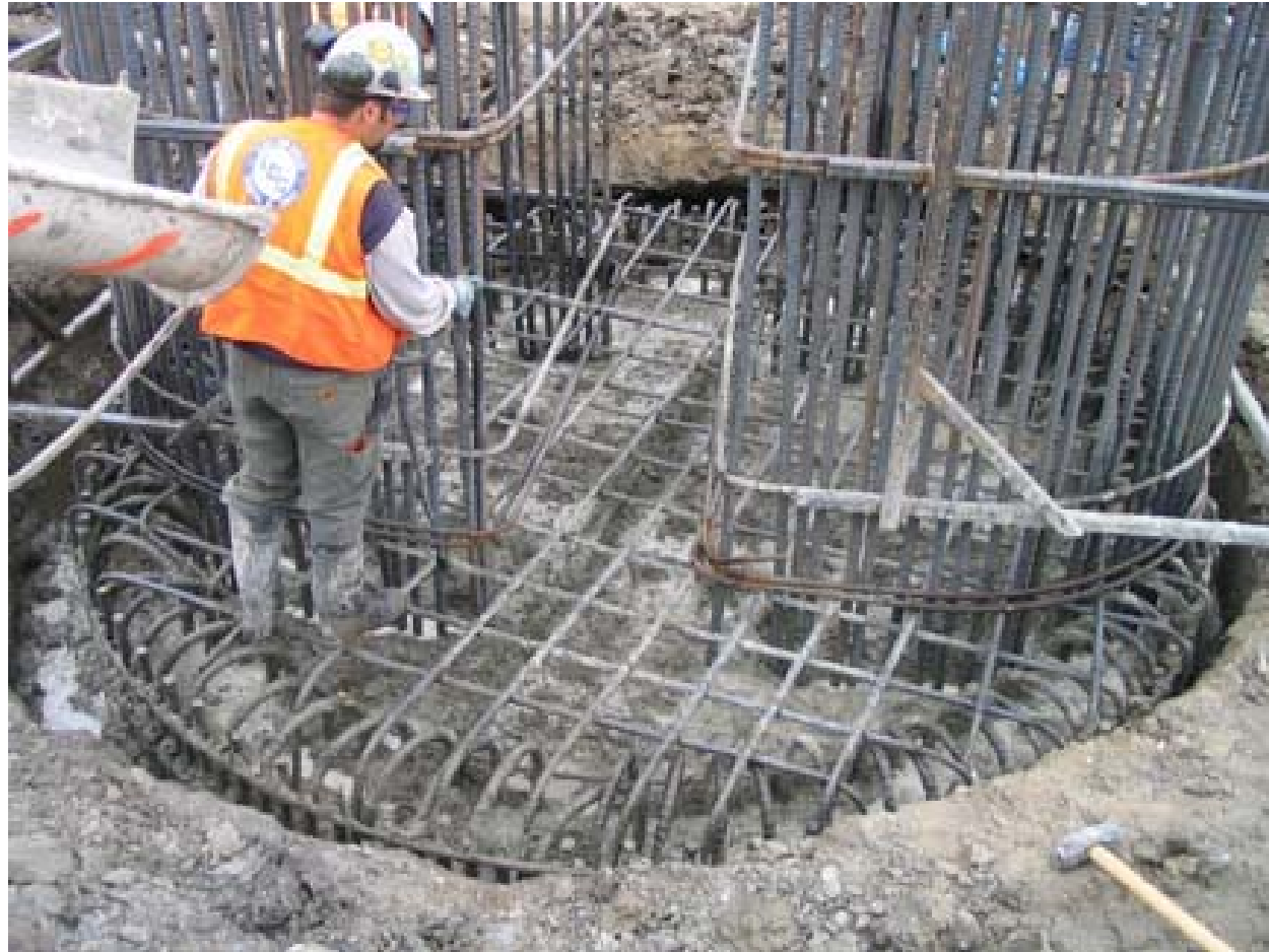
Figure 10: Dowels are Put in After The Pour When The Concrete is Still Fresh.
