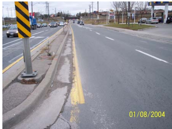
Figure 5 – Condition of microsurfacing after 11 years of service.
