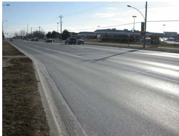
Figure 1 – Pavement surface on Thicksen Road in Whitby before microsurfacing application. The shine is due to the presence of polished stone in the surface course mix.
