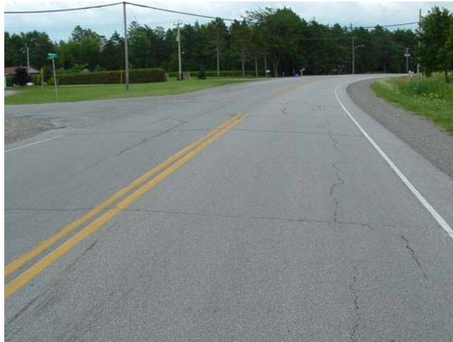
Figure 6 – Low to medium severity alligator cracking observed on the road.
