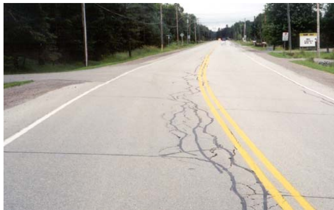
Figure 7 – Localized medium severity alligator cracking.
