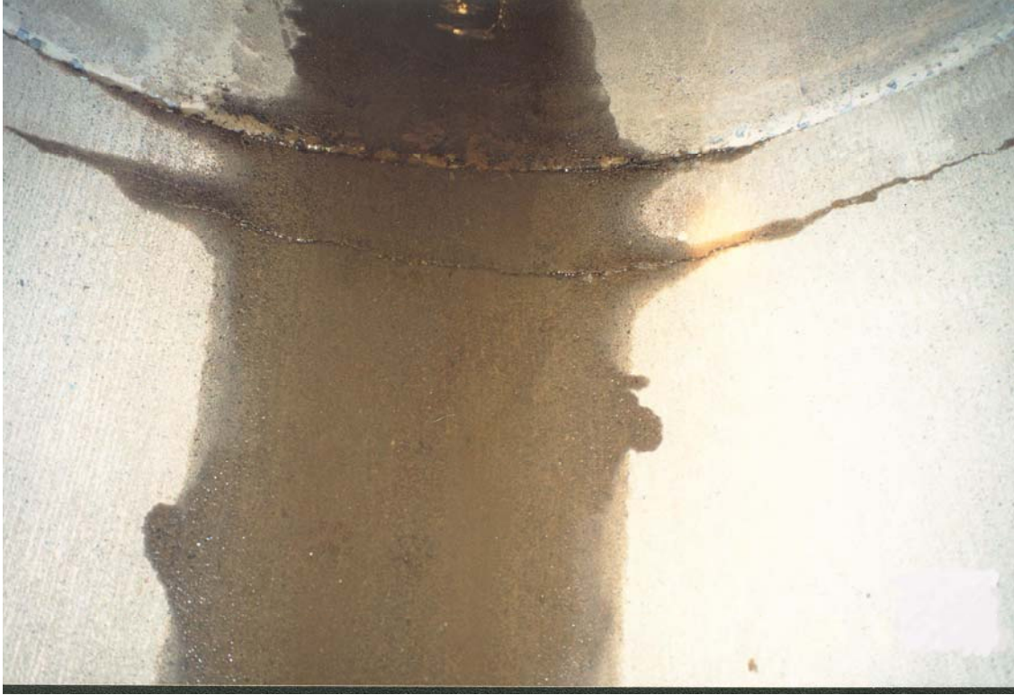
Figure 5 Typical circumferential cracking.
