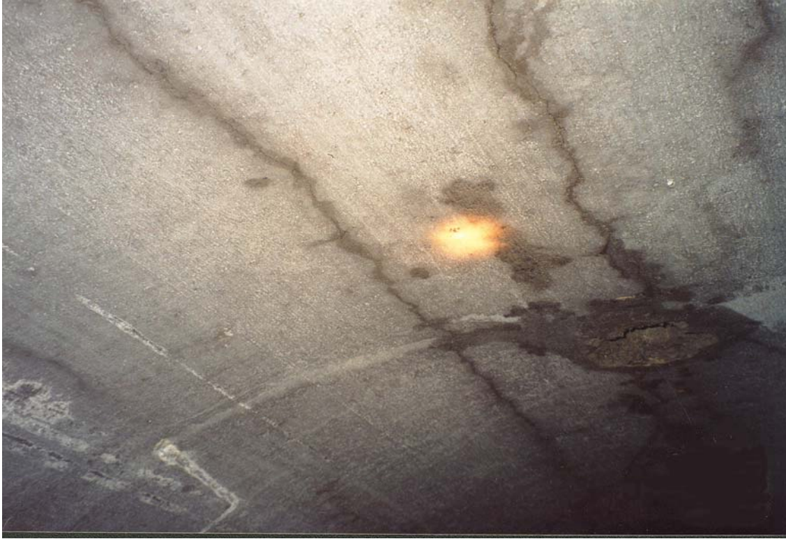
Figure 6 Longitudinal cracking observed in two installations out of 50.
