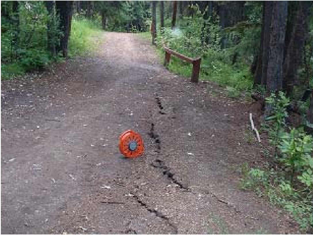
Figure 13 Tension cracks in the lower trail
